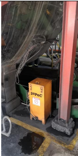
Dosing unit Boiler 3
