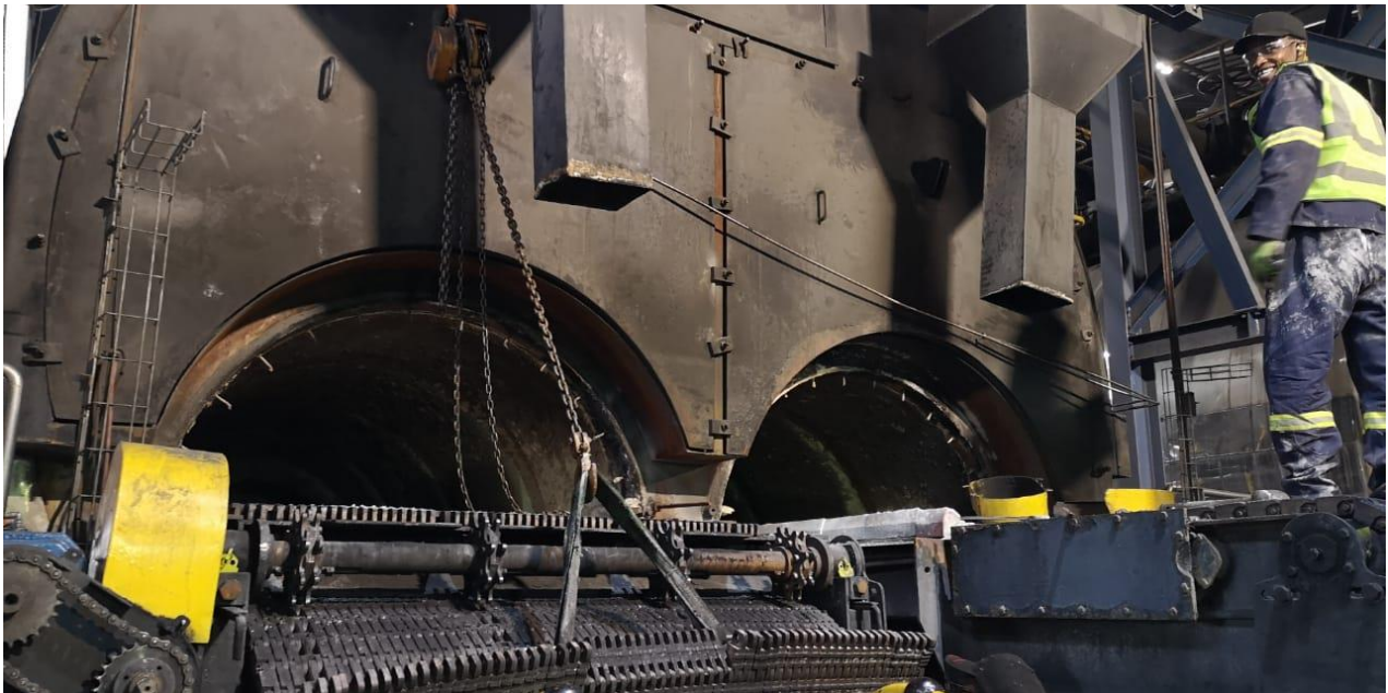
Front view of Boiler no 3
