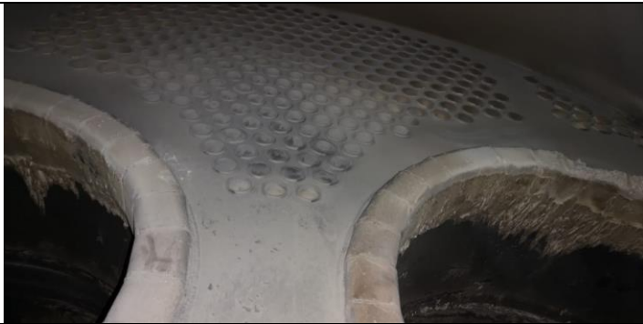
Reversal chamber Boiler 3
